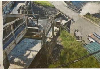
Water rushes through the log sluice at FirstLight's Cabot Generating Station in Montague. (DON TREGER / THE REPUBLICAN)
